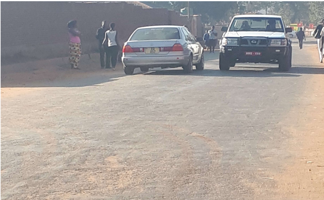
Photo 4.11.2 – Shows uneven road surfacing
