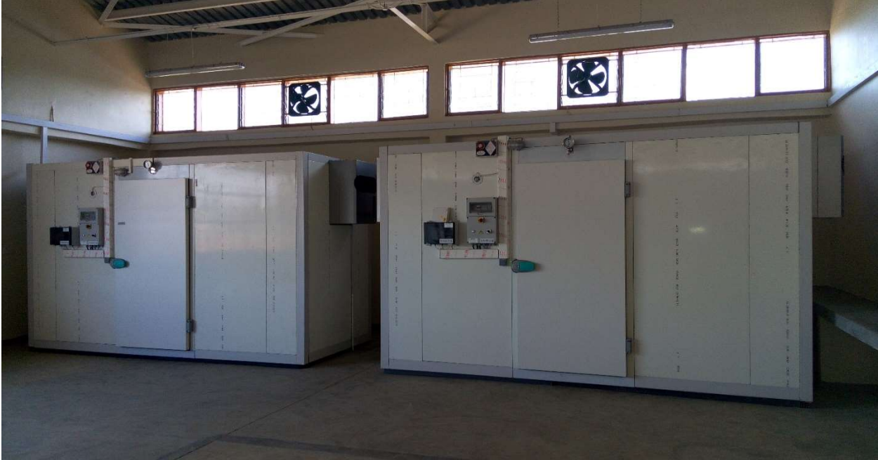
Picture 4.2.3.1 – Refrigeration Units in Cold Room
